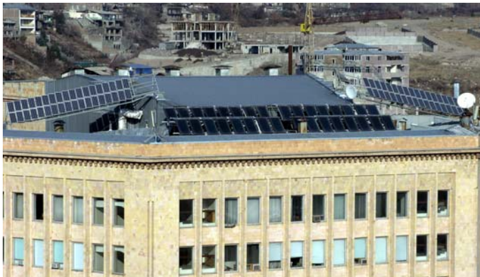
Solar panels on roof of AUA
